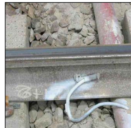
Be very careful of even small cables attached to a rail.
